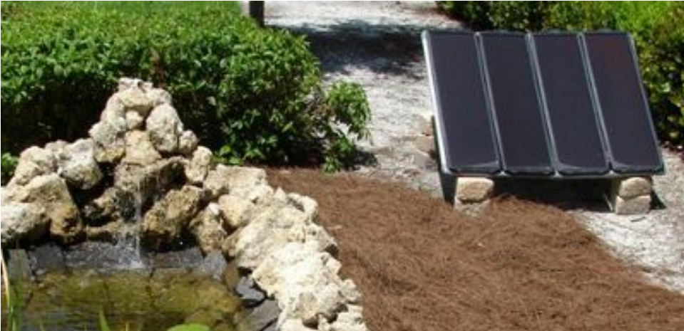
Figure 1: Solar panel array from kit providing power for water fall pump
